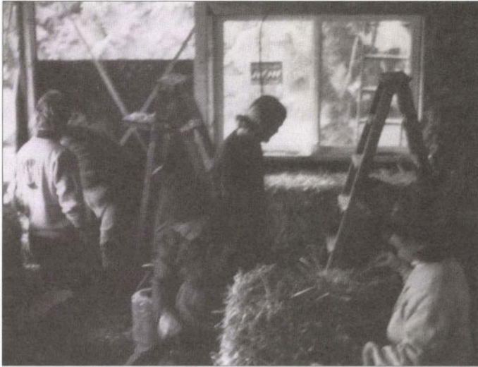
Building with straw bale—human-sized materials, and the direct use of human hands at a human-scale pace. Another home in Maxwellton Creek.
