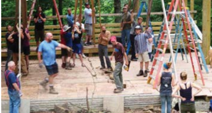
Our work afternoon involved supporting trusses on the roof over the amphitheater.
