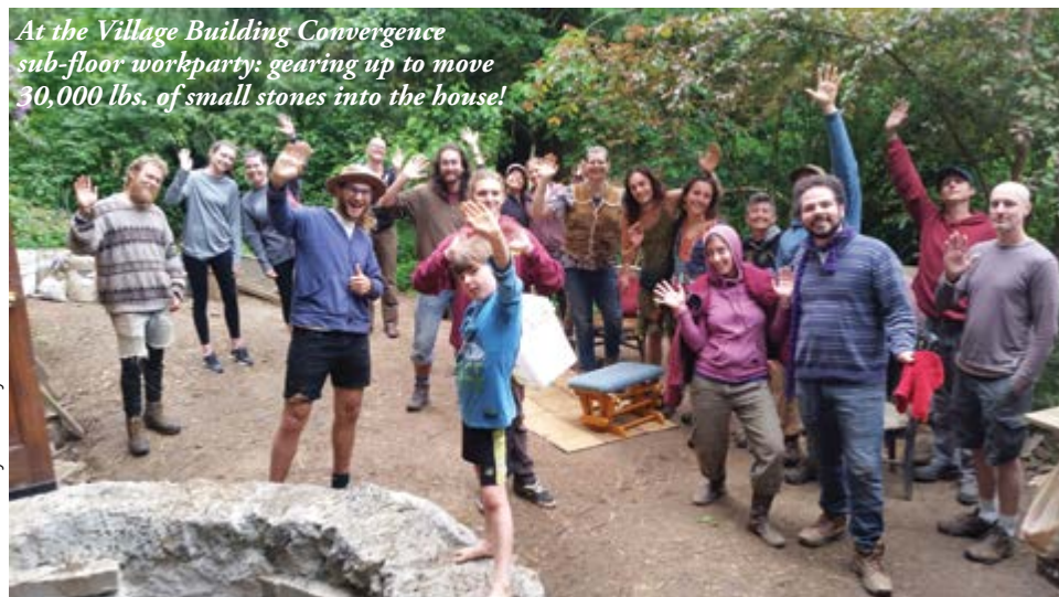
Workparty silliness and great teamwork, building the rough layer of the earthen floor.
