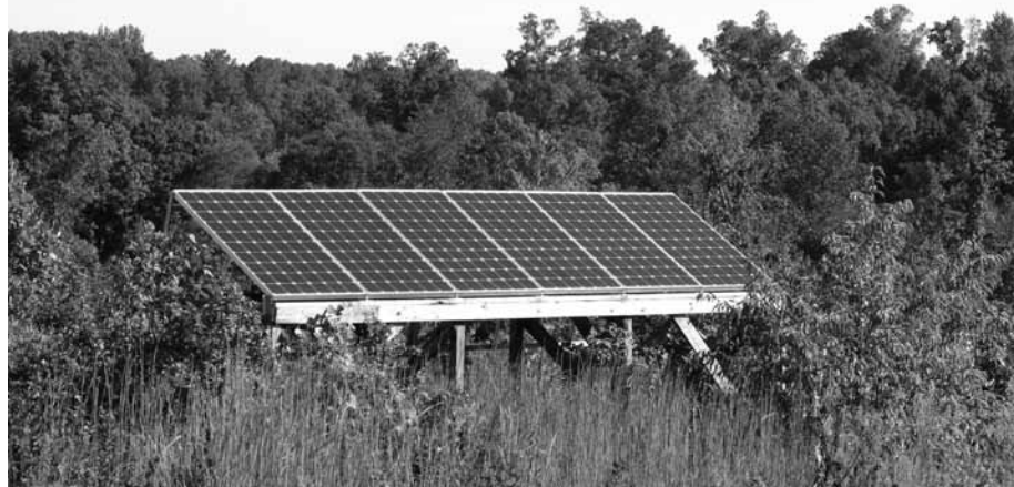
In summer, this 1400 watt array runs the main well pump. In winter, it powers blowers in the house that distribute solar radiant floor heat.
