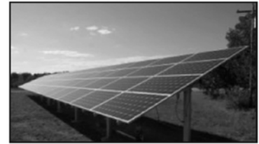
90KW in Solar Installations
