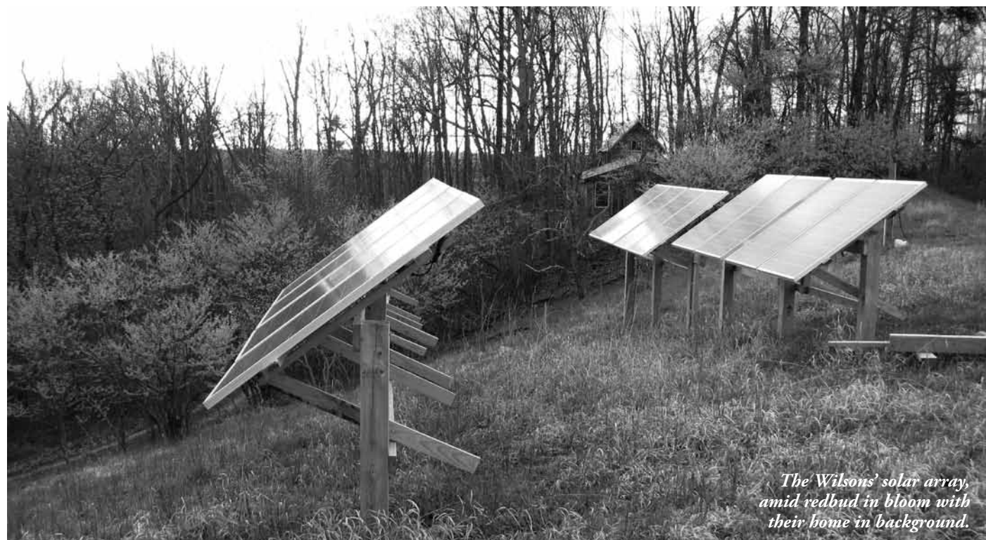
Close-up of treated wood framework for panels—easily adjustable for seasonal tilt.
