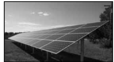
90KW in Solar Installations
