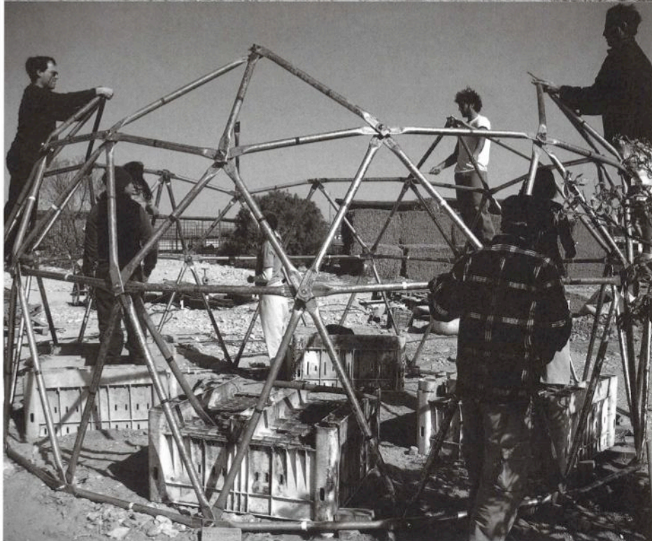
Top: The third dome frame is constructed next to the second one, onto which the first courses of strawbales have been tied. The bales are pre-plastered on both the interior and exterior faces. Bottom: Green Apprenticeship participants construct the earthquake-resilient geodesic frame that carries the weight of strawbales and earth plaster.
