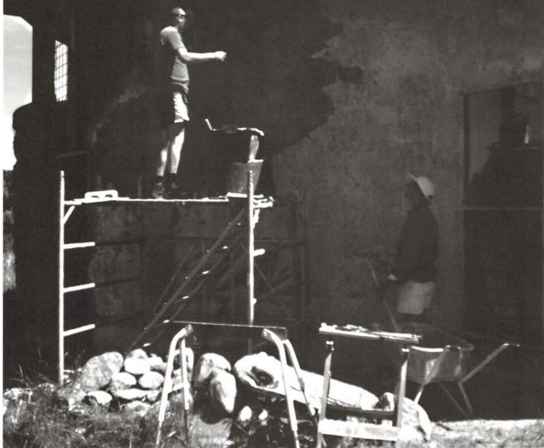
Jens Helt shows Niels how to throw lime plaster, giving the wall a professional touch.
