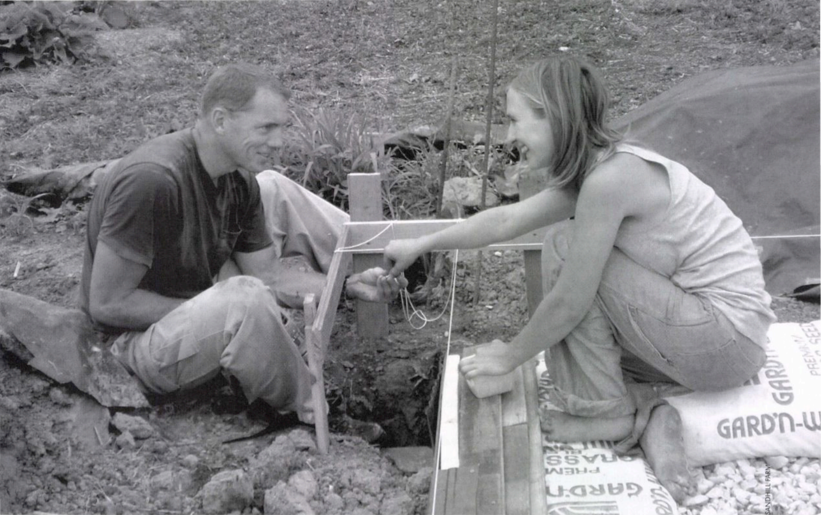
Sandhill members Greg and Steph build an earthbag foundation for the new community greenhouse.
