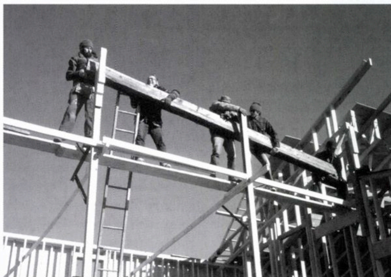
Raising a beam for the Bioshelter balcony roof, 1981; Bel Paulson in center.
