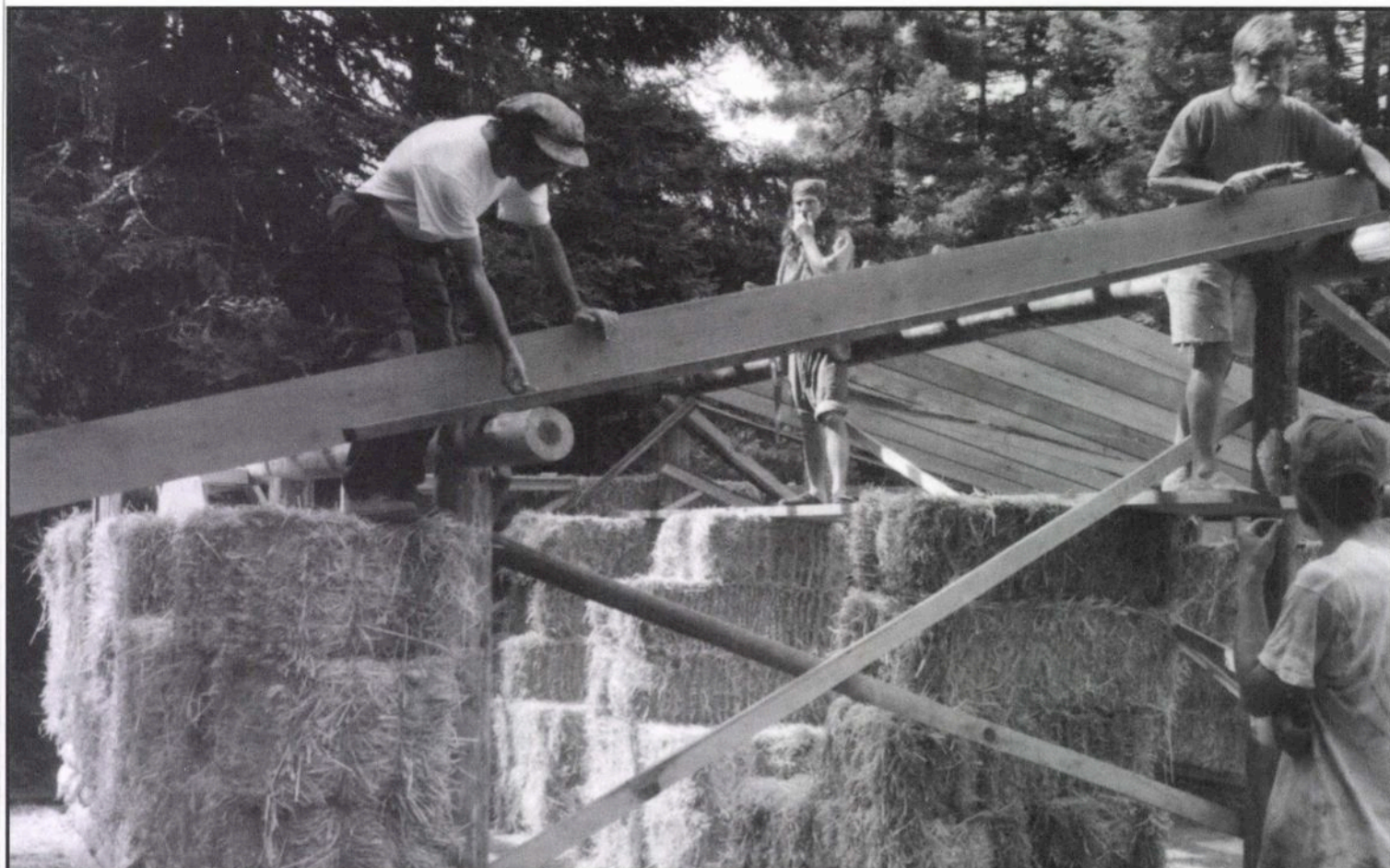
During one week-long work party, participants built the foundation, strawbale walls, roof beams and rafters of this 400 sq. ft. cabin.
