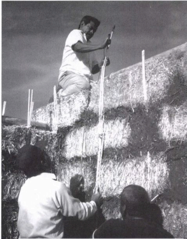
Using "exterior pinning" like this works far better than interior pins to stabilize bale walls, and is rapidly becoming the preferred method worldwide.
