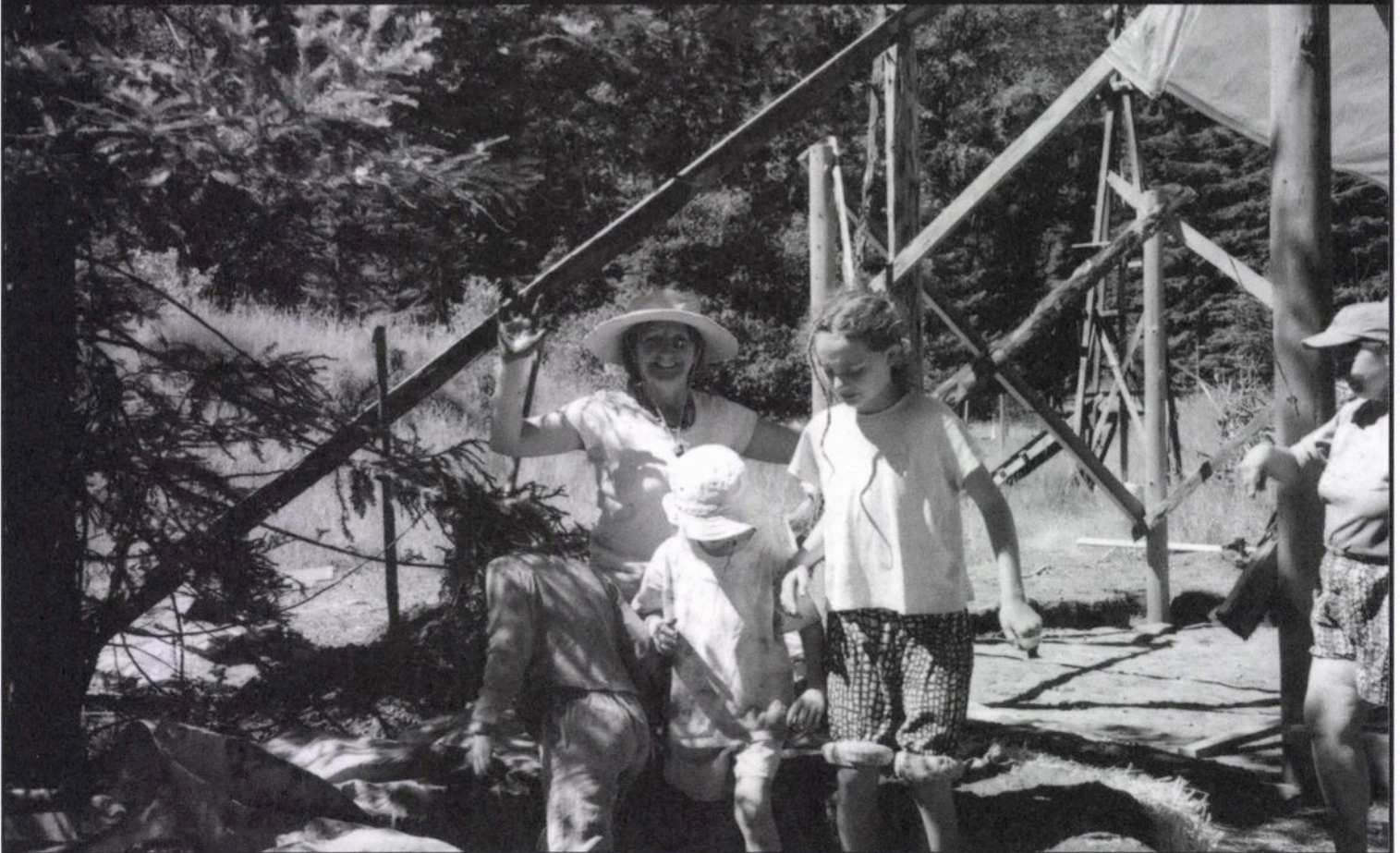
Everyone loves to play in the mud. Children at a work party help mix clay, sand, straw, and water for an adobe floor.
