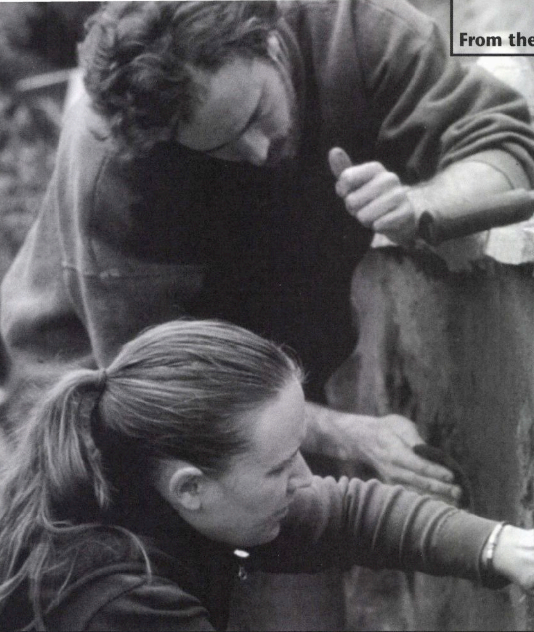
Robert Bolman, above, leads crew on structural cob wall and community information kiosk during Portland's Natural Building Convergence.
