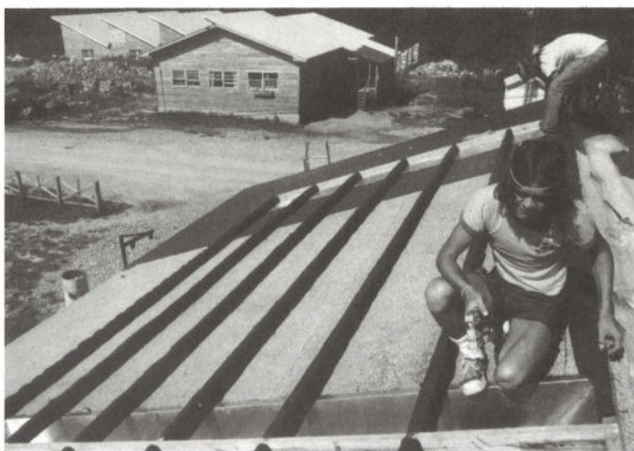
Peter Barger installs an active solar heating system on a Farm roof, c. 1976.
