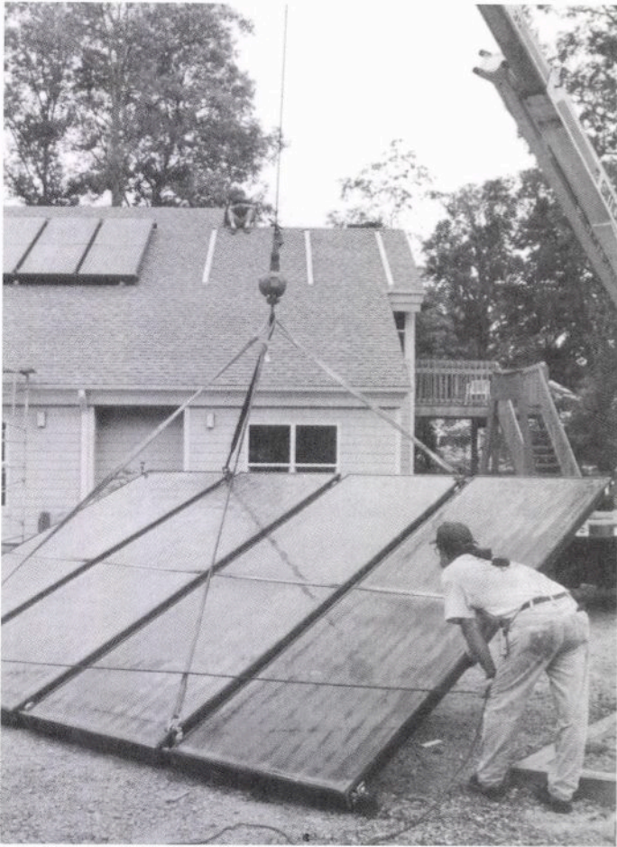
Westwood interiors are centrally heated by a combination of active solar and natural gas. The last solar panels are installed on common house roof, 1998.
