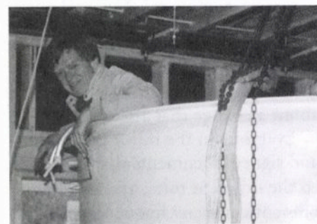
Central heating, cooling, power, and communication systems were designed by Bill Fleming, here installing the solar heat collection tank in common house basement.
