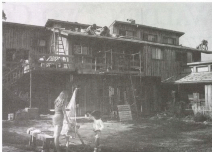
Roofing the new building at Twin Oaks. “We went into it, head over heels, with very little planning or investigation,” says cofounder Kat Kinkade.
